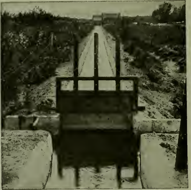
Sluice-gates in California.
